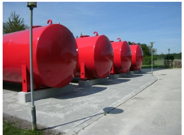
4 x 100 m 3 tanks diameter 2900 mm
